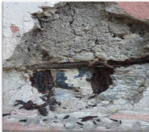
Fig.6. Corrosion in column reinforcement
