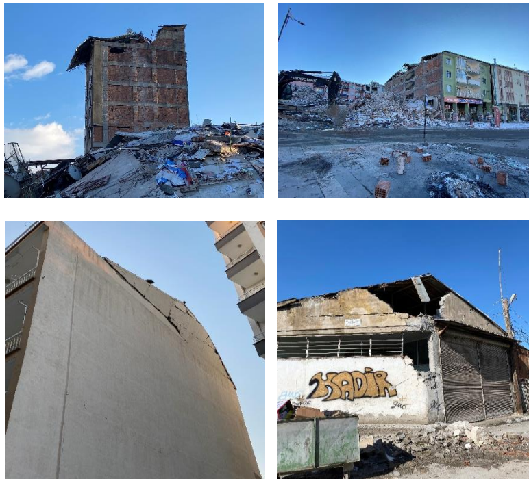
Figure 8. Failures of gable walls in Malatya [10]
