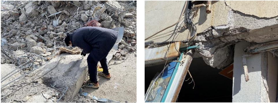
Figure 13. Poor quality of materials [10]
