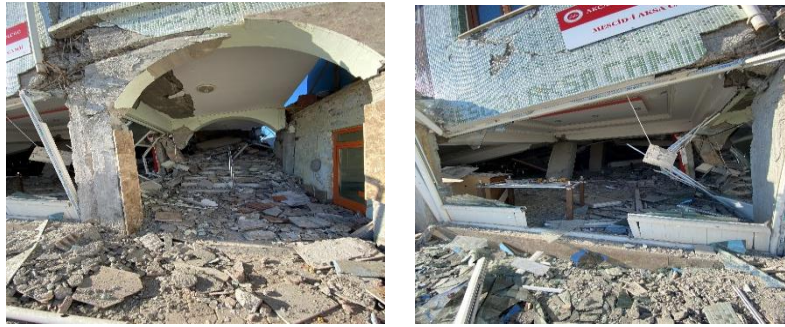
Figure 7. Examples of damage due to soft storey [9]
