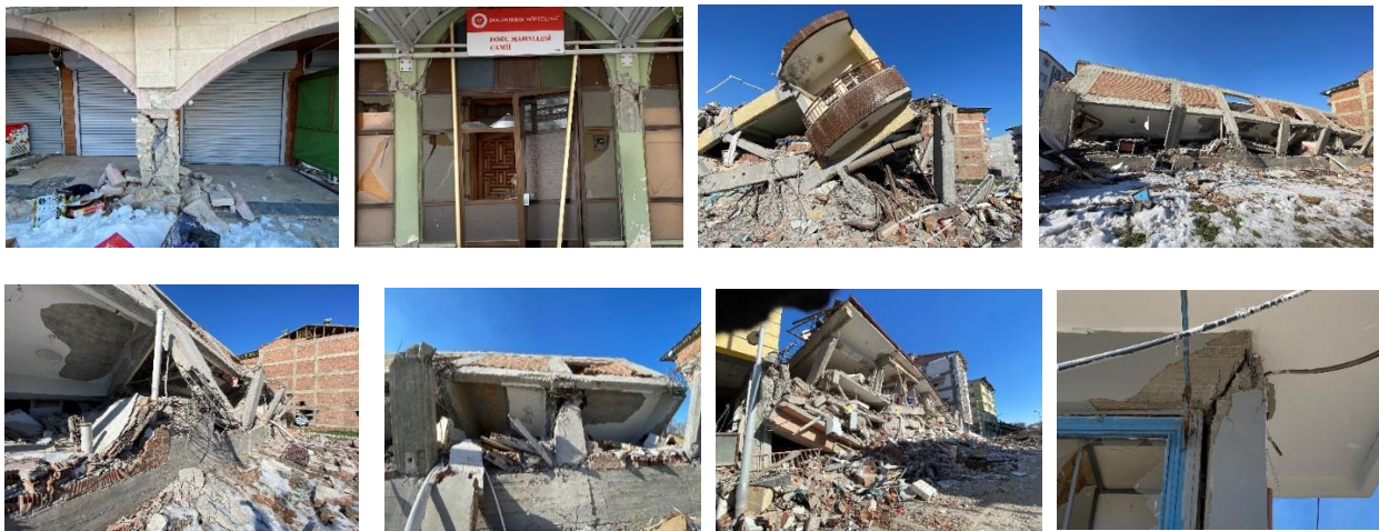
Figure 10. Damages caused by inadequate reinforcement [10]
