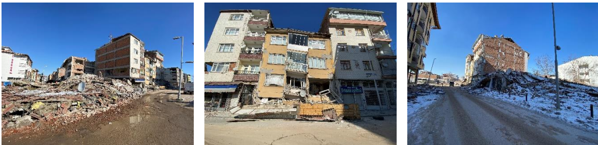
Figure 11. Examples of damage and collapse in adjacent structures [10]
