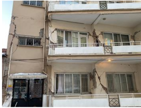
Figure 14. A masonry structure with a corner failure mechanism and shear cracks (38.35371 N, 38.32353 E) [17]
