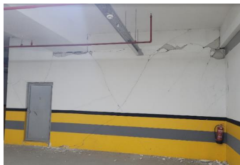
Figure 5. Infill walls at the isolator (parking) story, constraining the movement of the isolated superstructure [10]
