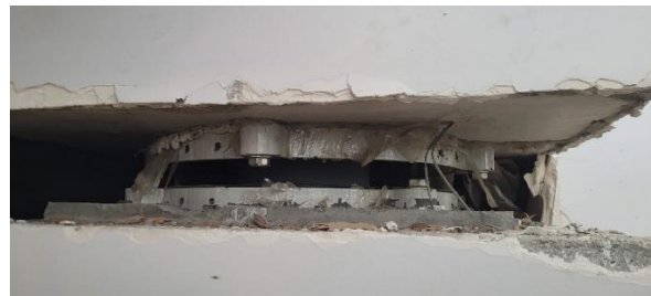
Figure 2. One of the friction pendulum type seismic isolators of Elbistan State Hospital [10]
