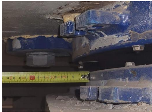
Figure 10. Residual isolator displacement in Osmaniye State Hospital [12]
