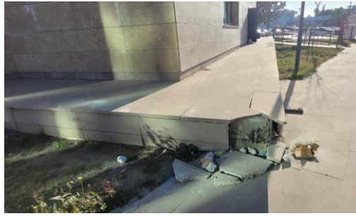
Figure 9. Minor collision damage between a corner of the isolated structure and the pavement [11]
