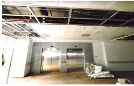
Figure 12. Flood damage at upper stories of isolated superstructure and resulting red (rust) residue at Osmaniye State Hospital [12]
