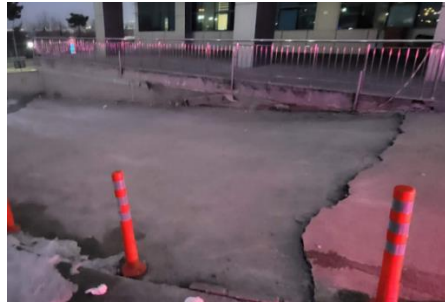
Figure 6. The access ramps of the hospital building cracked and deformed in places where the seismic gap would have been [11]
