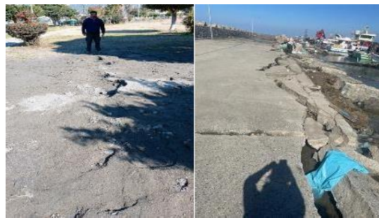
Figure 10. Surface manifestations of the sand boil as seismic liquefaction in Iskenderun Hatay (left), lateral spread due to liquefaction in the fishing harbor area in Iskenderun, Hatay (right) [19]
