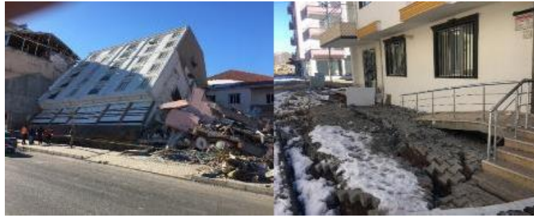
Figure 6. Tilting of buildings and heaving of soils around foundations due to liq-uefaction (Adiyaman- Golbasi) [19]
