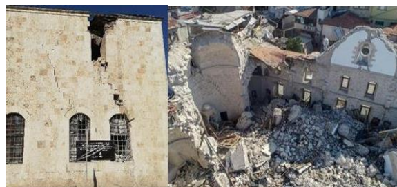
Figure 13. Damaged historical structures in Antakya after earthquake sequence; a) Habib-i Neccar Mosque (courtesy of the EEAT), b) Rum Orthodox Church [19]
