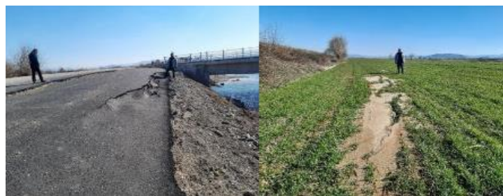
Figure 11. a) Lateral spreading (left), b) sand boiling due to soil liquefaction (right) [19]
