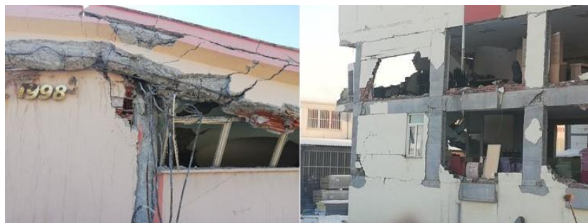
Figure 15. Structural deficiencies observed in damaged buildings (courtesy of the EEAT) [19]
