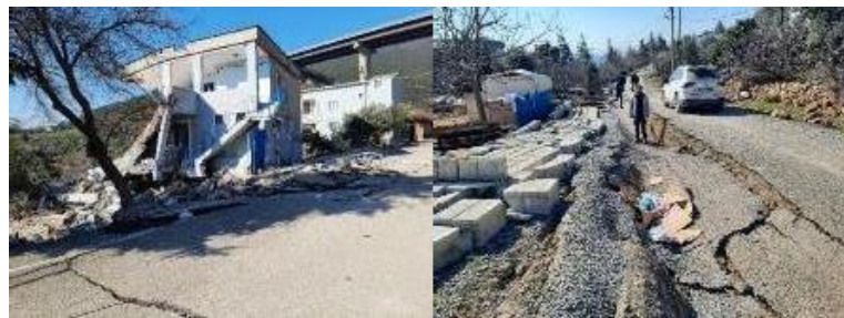
Figure 7. a) Major damage to houses due to surface faulting (left), b) deformations and settlements due to surface faulting on the road in Nurdagi (right) [19]
