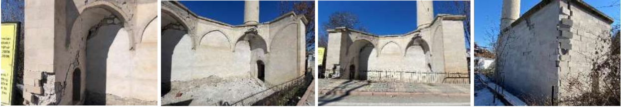
Figure 11. Damage distribution of Sütlu Minare Cami [10]
