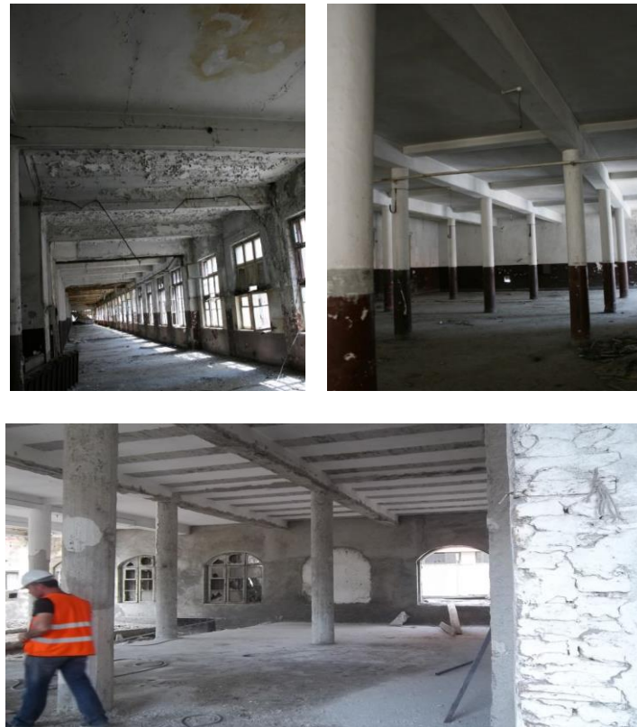
Figure 21. a) Condition of B2-Block before CFRP repair and strengthening application; b) Preparation of the elements to be repair and strengthening in block B2; c) Preparation of the elements to be repair and strengthened in block B2 (Kasimzade Archive)
