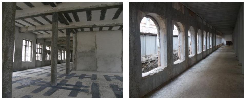
Figure 22. a) Column beam and floor repair and strengthening with CFRP Fabric in B2 Block; b) Masonry walls repair and strengthening in B2 Block (Kasimzade Archive)
