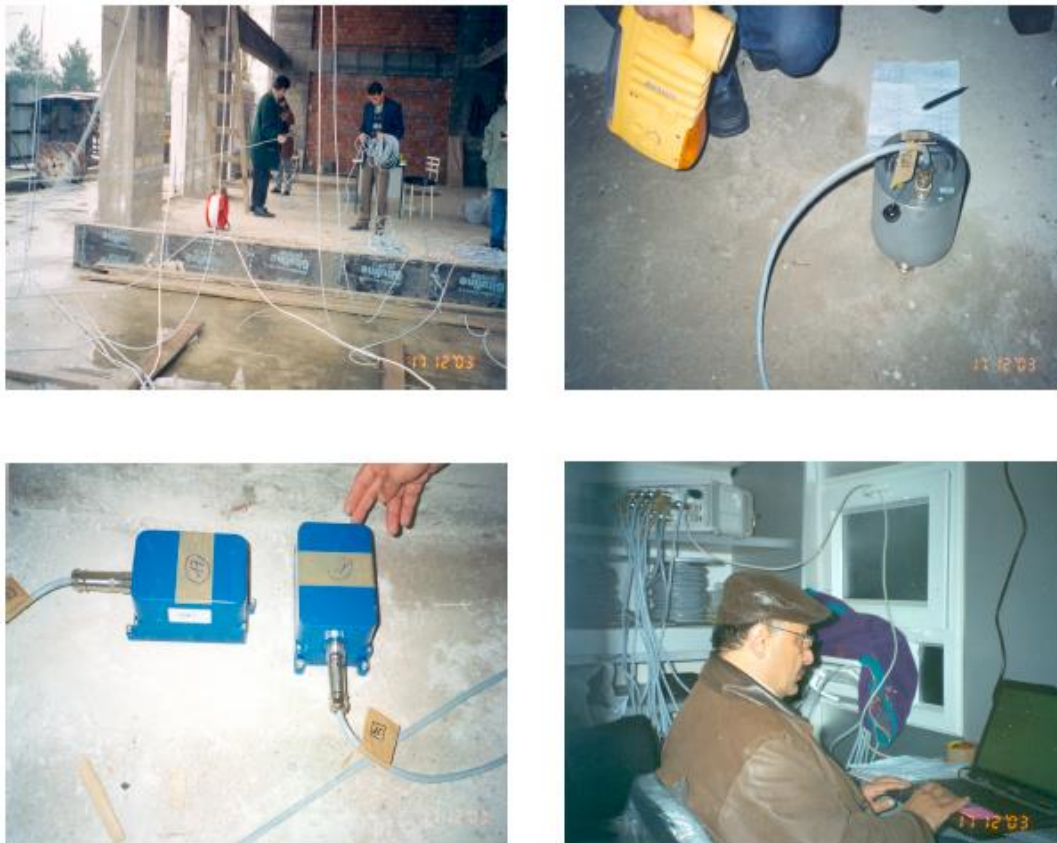
Figure 3. Installation details of devices (accelerometers) on the 1-11 floors, seismometer on the ground floor, checking the operability of devices on the computer respectively (Kasimzade Archive)
