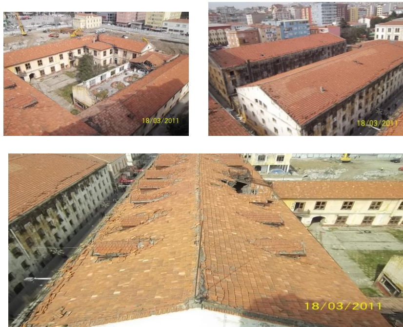
Figure 19. A-block view before repair and strengthening; b. C and D-block view before repair and strengthening; c. B block view before repair and strengthening (Kasimzade Archive)
