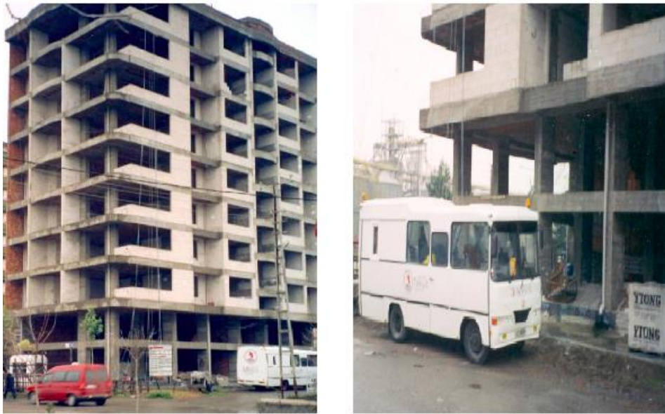
Figure 2. Experimental (real) model of structure and layout of the devices (accelerometers) on it (Kasimzade Archive)
