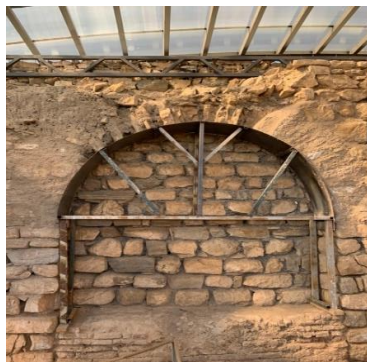
Figure 19. Consolidation of an Arch in order to preserve and present the Architectural assets,
