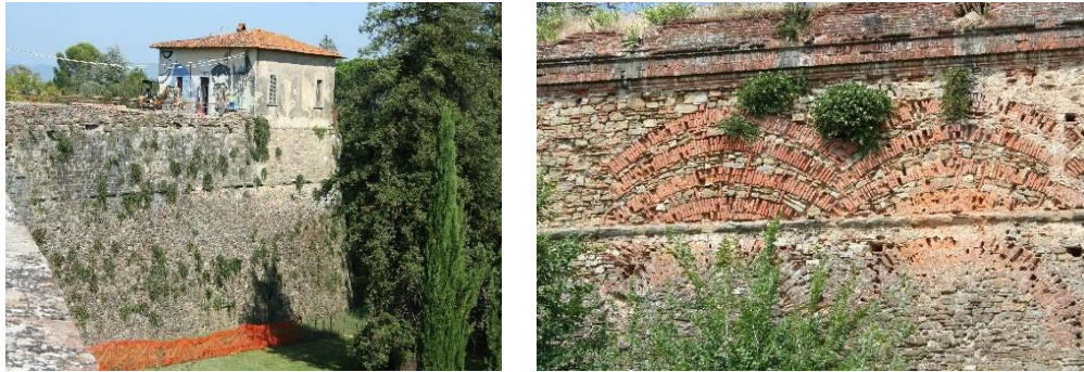
Figure 3, 4. The Fortress before the exterior walls restoration project
