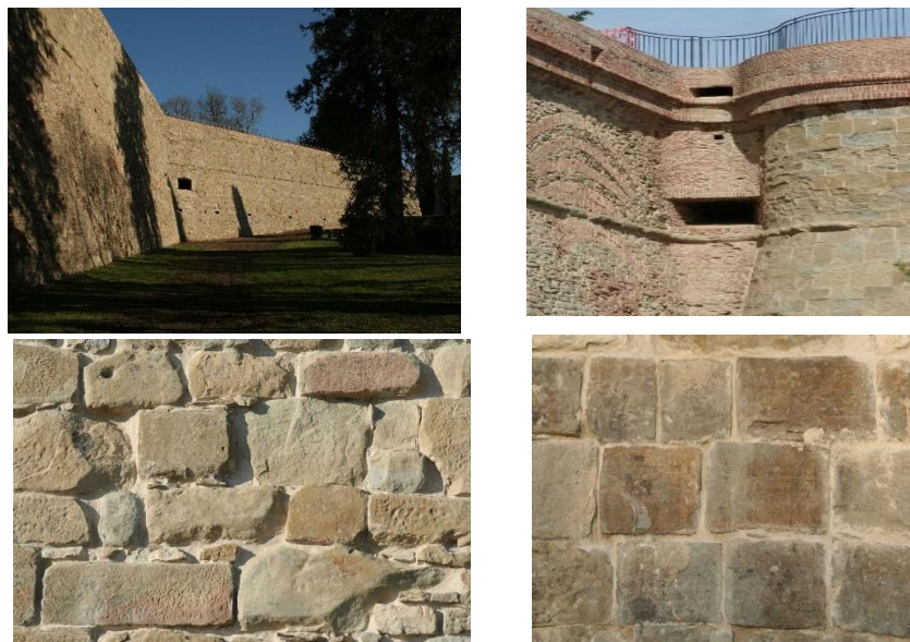
Figure 15, 16, 17, 18. The Fortress after the restoration of the external walls and details (end of phase one)
